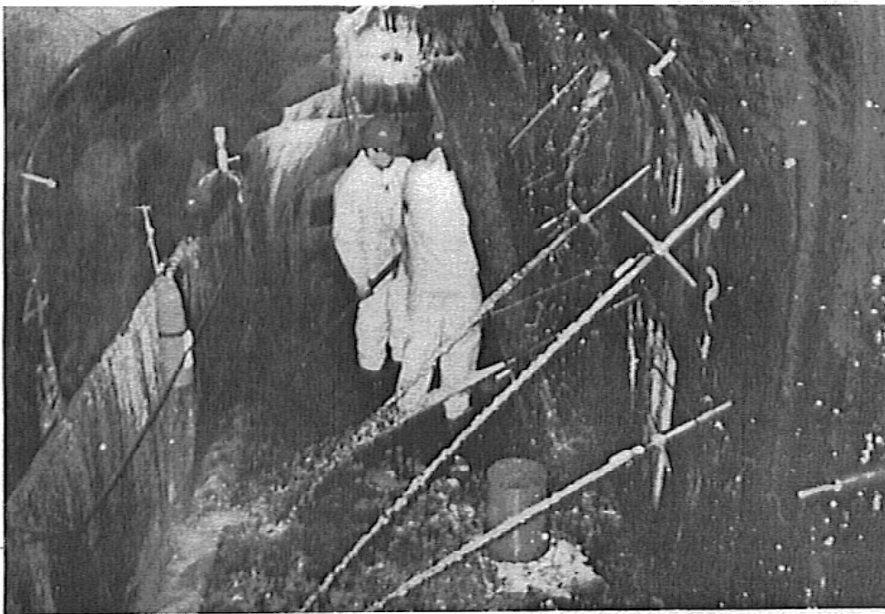
Holes drilled upstream of the lower gallery of the Santeetlah Dam intercepted individual flows of up to 400 liters per minute at full hydrostatic head seeping through joints. The fissures intercepted by the holes were subsequently sealed with epoxy resin using the RODUR system.
